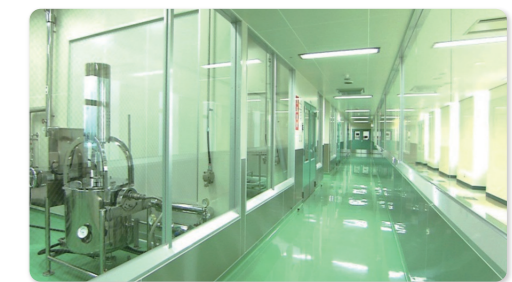
One machine per room to prevent cross-contamination.
